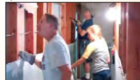
From left: Myron Hanke, from Church of the Good Shepherd, Vienna, Va.; Jill Durbin, Antioch (Tenn.) UMC; and Mark Dalhoff, Perritte UMC, Nacogdoches, Texas, install new wall board in a Houston home.
