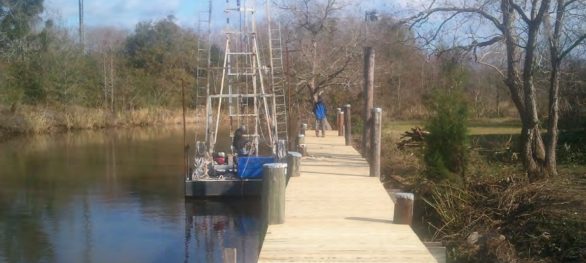
Tripp's completed Eagle project provides safer footing for people using the 110-foot pier for the Mobile Sail and Power Squadron.
