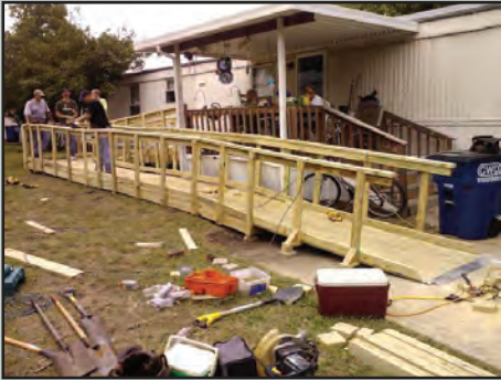
Men of Wylie UMC build a handicap ramp—one of six built in 2014.
