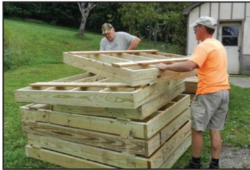
The ramps are built as modules so when a ramp is no longer required, the ministry can move it to another site.
